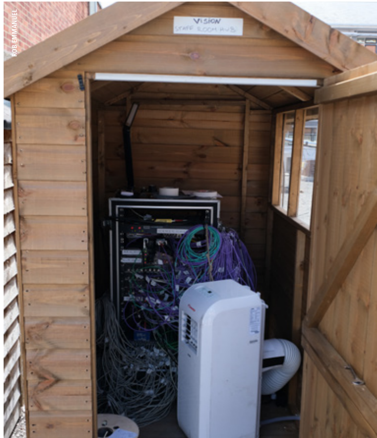
A&E's 'Staff Room' vision shed, housing the conversion equipment for 78 cameras, erected on the roof of the hospital
